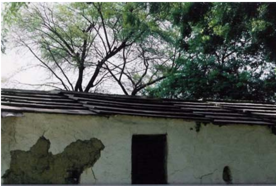
Building Construction. Fig. 15 Roof with a stone slab (Rajasthan, India) (photo by the author).
